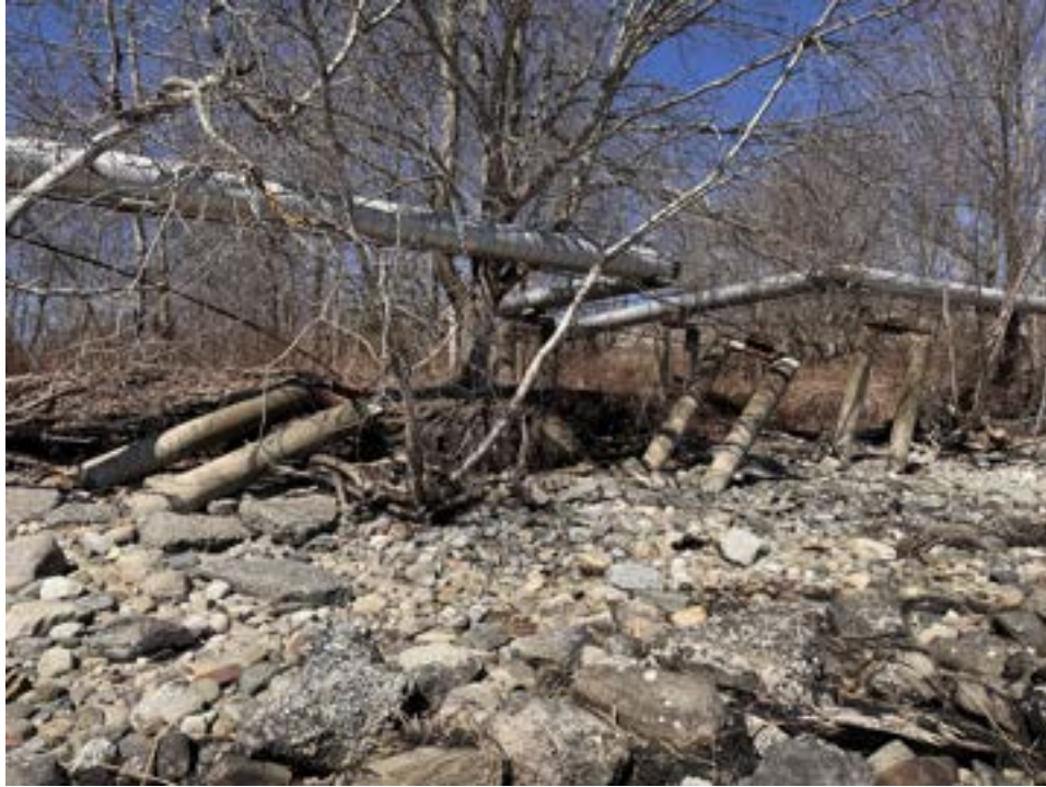
Photo #18 inactive & collapsing industrial pipe
