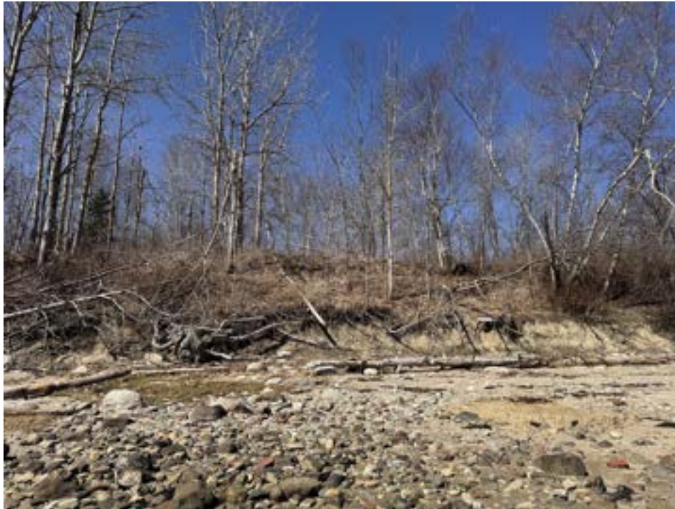
Photo #28 toe erosion on vegetated bluff
