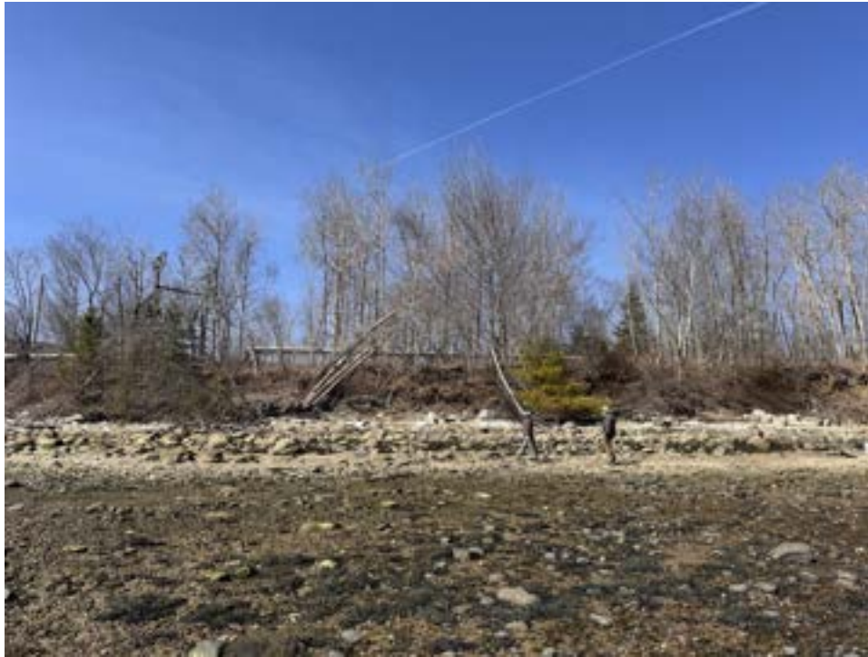
Photo #24 unstable vegetated bluff, inactive industrial pipe. 44.46601° N, 68.87790° W
