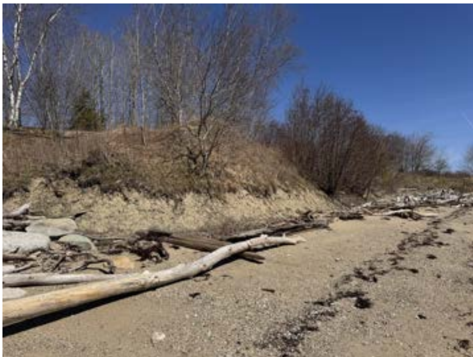
Photo #31 toe erosion on vegetated bluff
