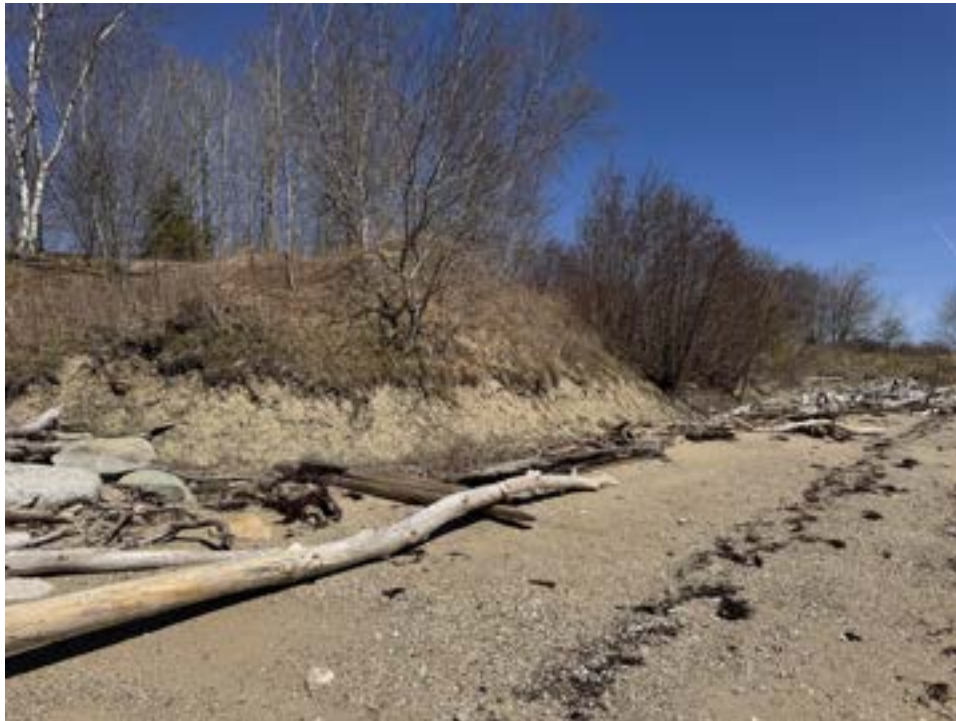
Photo #29 toe erosion on vegetated bluff
