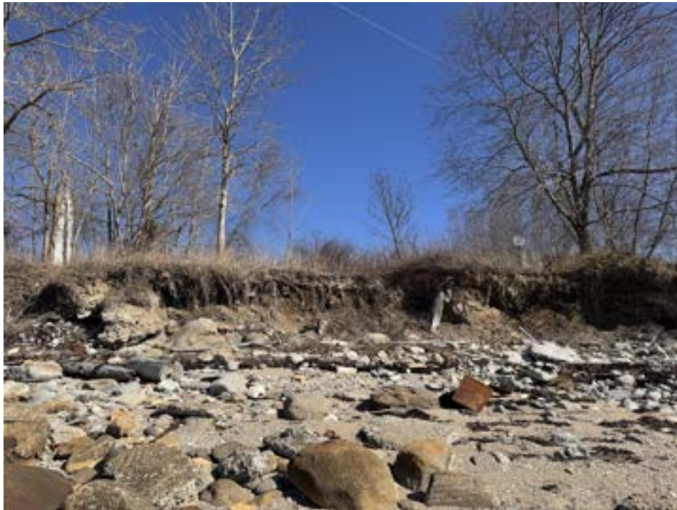
Photo #2. Highly unstable bluff, metal and concrete waste. 44.46480° N, 68.88035° W
