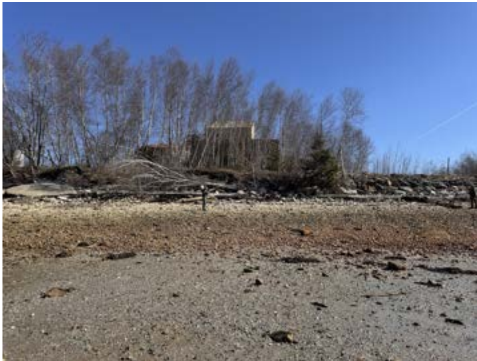
Photo #5. Discolored intertidal sediment, concrete, failed riprap, newly installed riprap 44.46468° N, 68.88003° W
