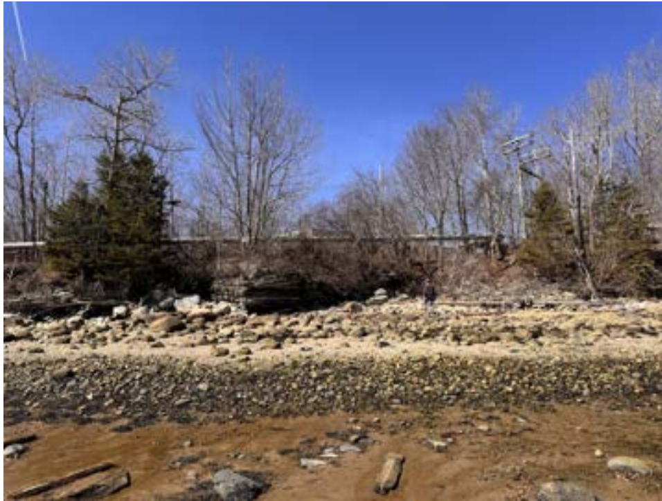
Photo #22 exposed demolition debris, inactive industrial pipe. 44.46571° N, 68.87799° W
