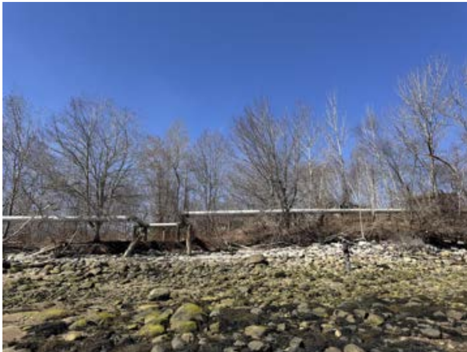
Photo #19 unstable bluff, inactive industrial pipe, unstable riprap 44.46528° N, 68.87786° W
