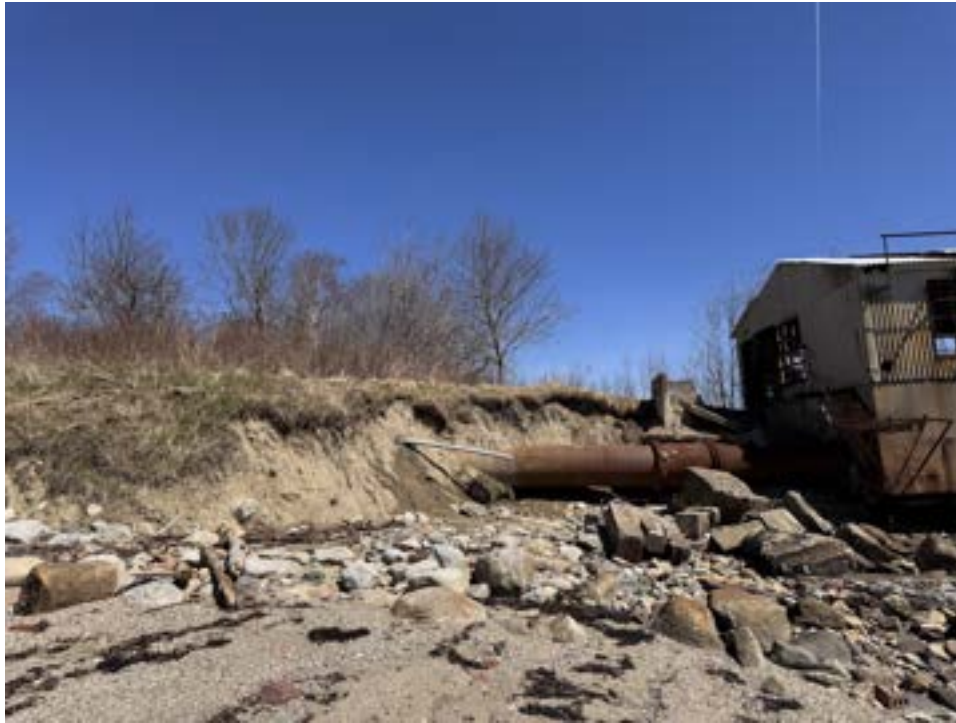
Photo #32 unstable bluff, abandoned building.
