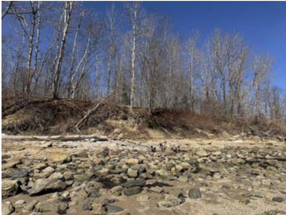
Photo #25 toe erosion on vegetated bluff
