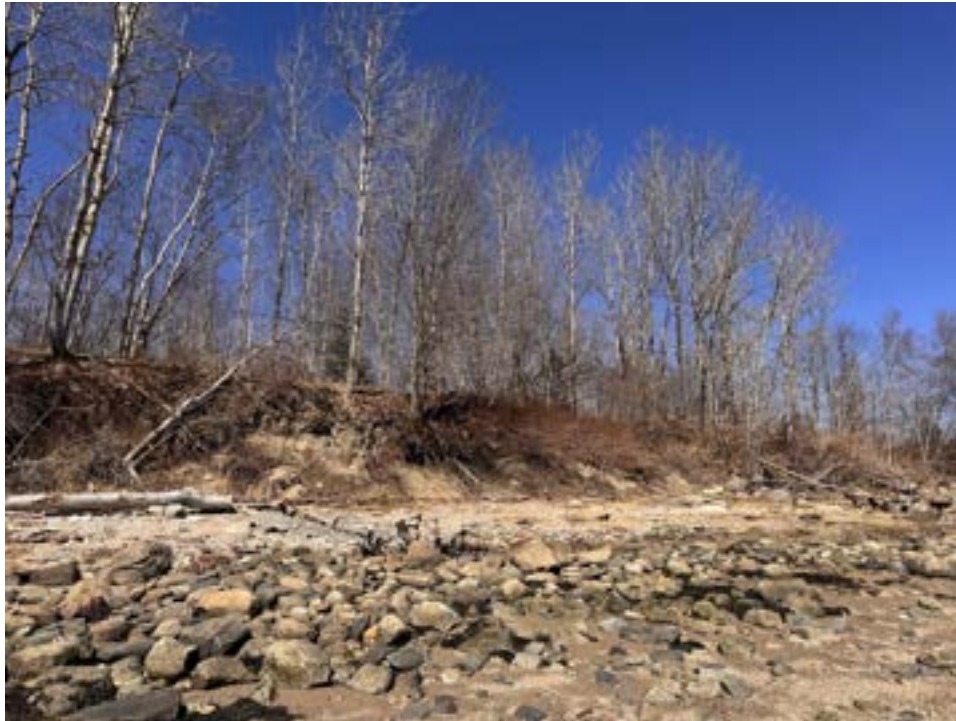
Photo #26 toe erosion on vegetated bluff
